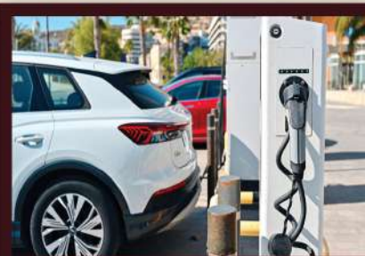
EV CHARGING POINT
