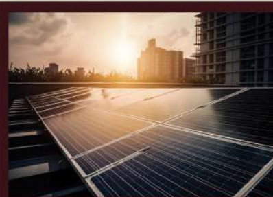
SOLAR PANELS FOR COMON AREA
